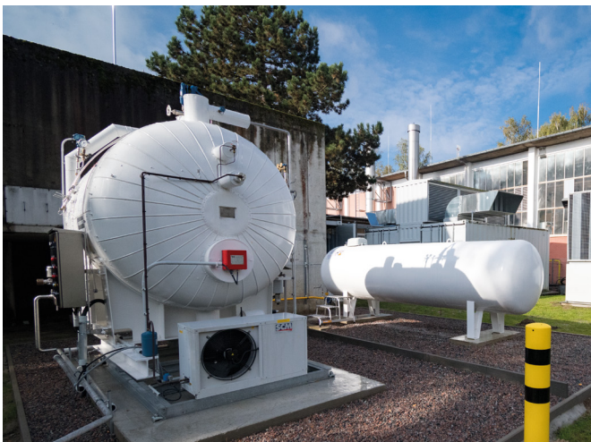
▲ Gas storage tanks for gas mixing facility
